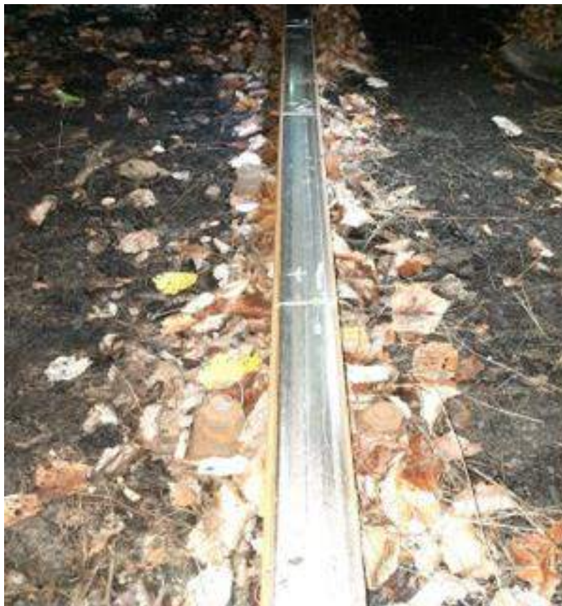
Image no. 9 – Technical condition of the line in the area where the accident occurred
