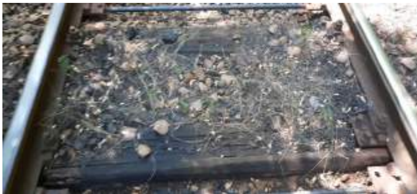
Photo no.11 (dated 16.07.2024) - Sleepers and anchoring rods on the curve where the railway accident occurred
